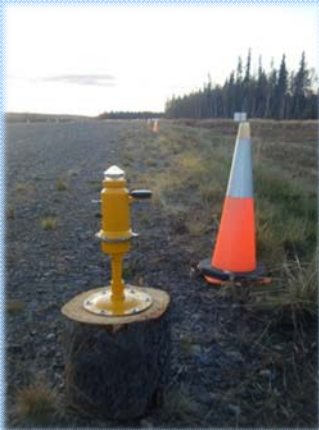
LED Lights that mark the corners of the Napaimute Airfield
